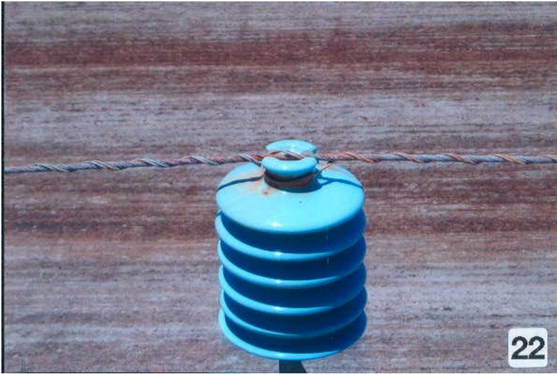
Photograph of Aerial Pole D250/16/6 Insulator and Conductor Tie
