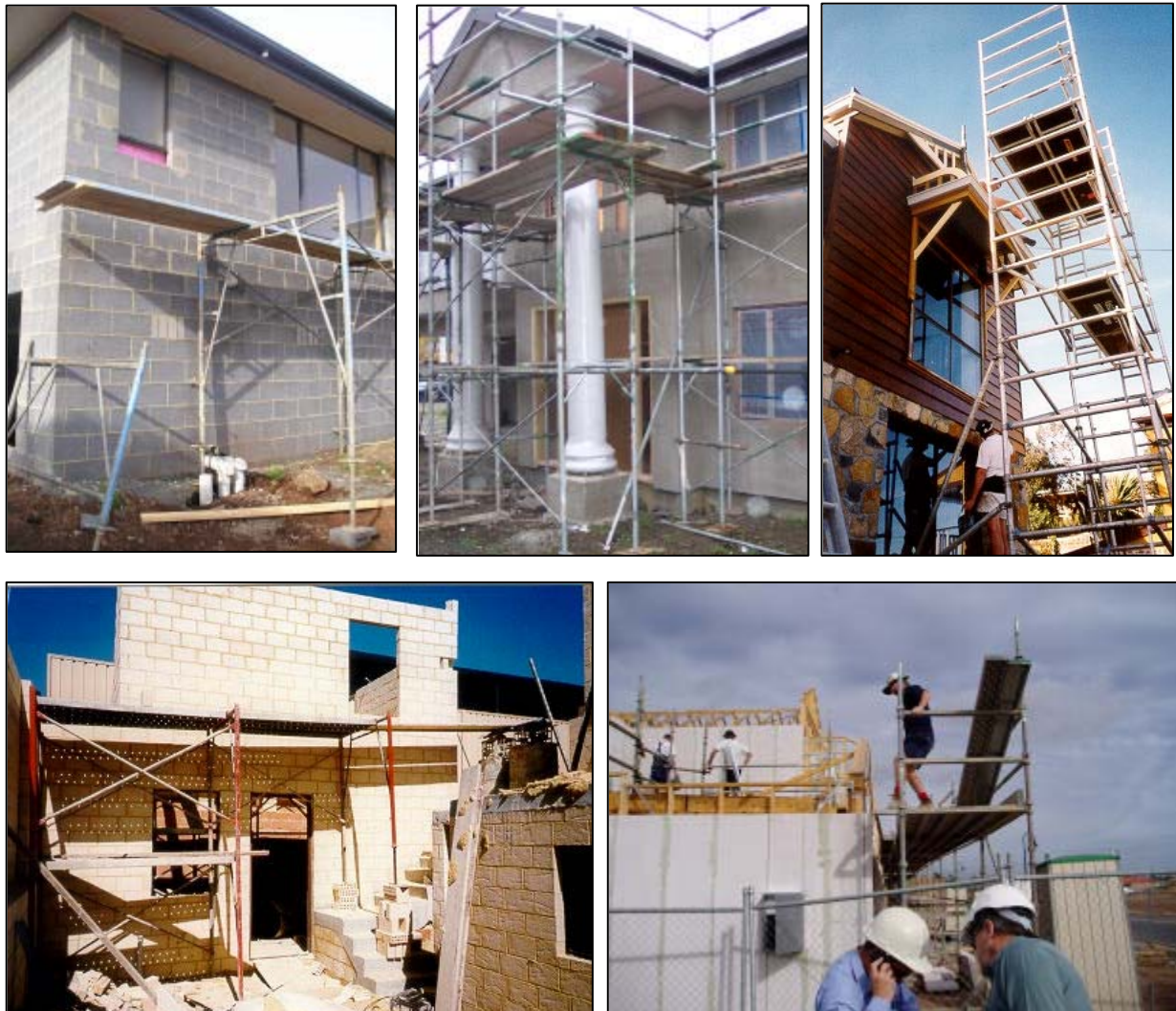
A selection of scaffolding “shockers” encountered by inspectors during the project. Top, from left, shockers seen in Tasmania, New Zealand and Western Australia. Above left, a shocker in Western Australia and, above right, one in South Australia.
