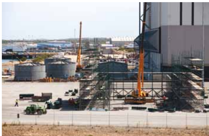
Cimeco has erected an enclosure at the CUF to blast and paint tanks for its new workshop.
