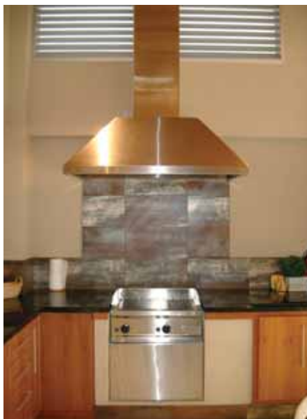
A commercial gas barbecue with mechanical ventilation.
