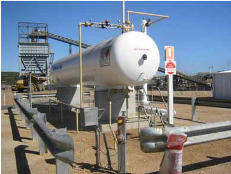
On-site LP Gas storage
